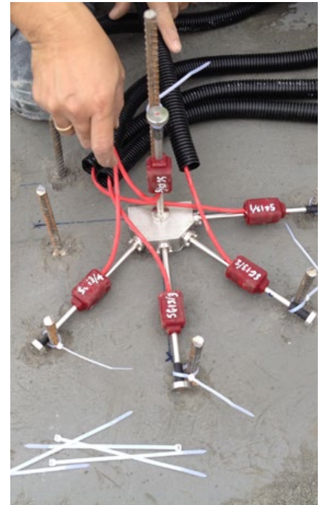
WW Strain gauges installed in special rosette configuration - Ulu Jelay Dam
