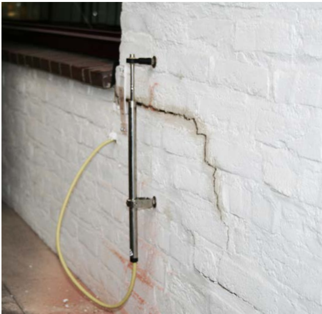
Displacement transducer for crack monitoring
