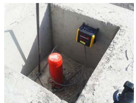
Sisgeo Mini-OMNIALog datalogger mounted to the side of the manhole
