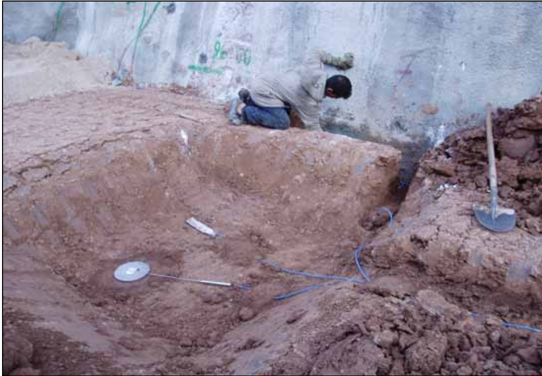
Positioning of the instrument's cables
