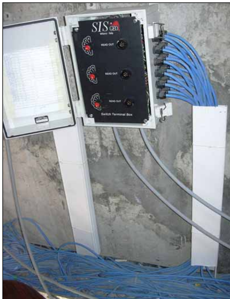
Switch measuring box for manual readings
