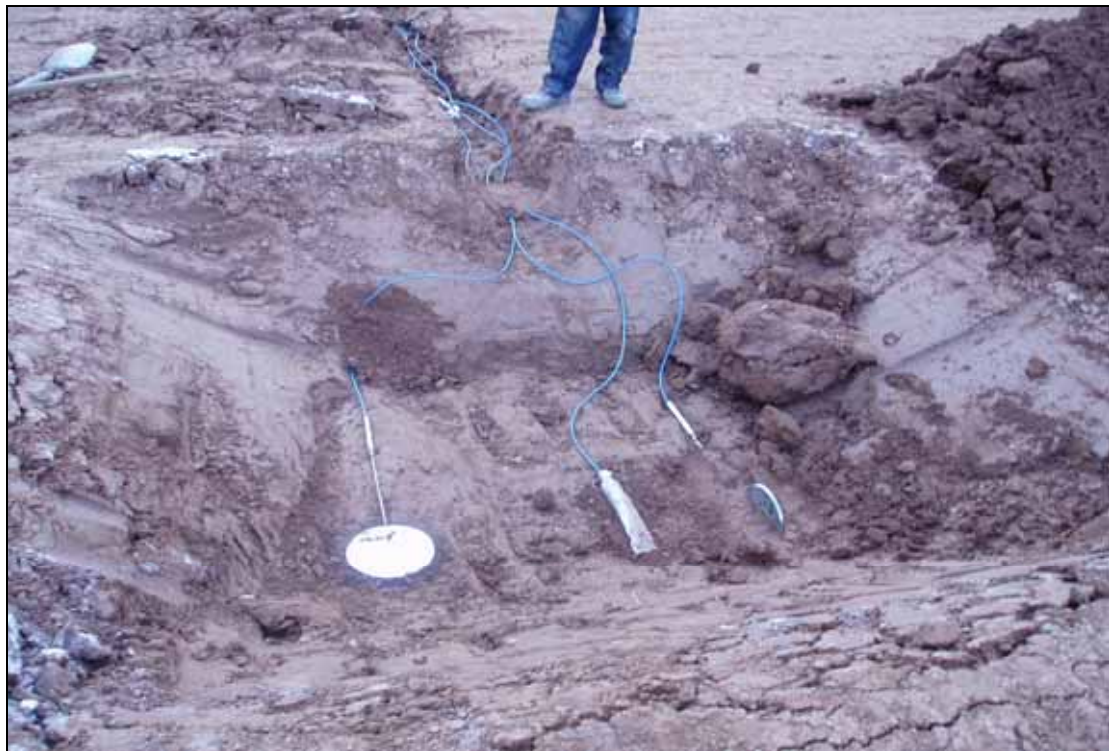
Installation of earth pressure cells in two direction and pore pressure transducer
