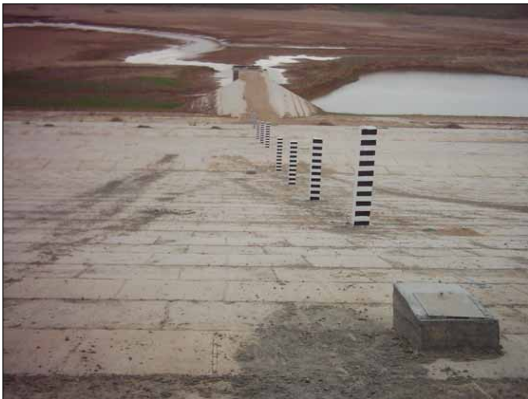
Staff gauges for direct readings of reservoir level
