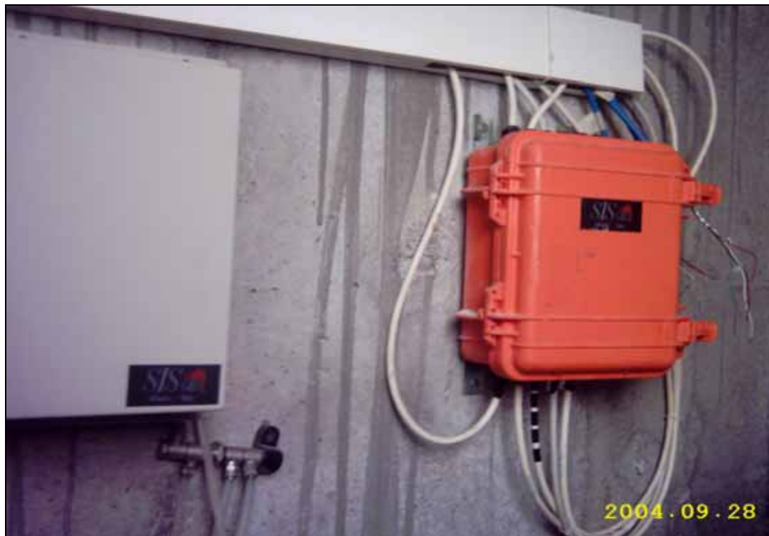
DSM reference point (left) and switch measuring box (right)
