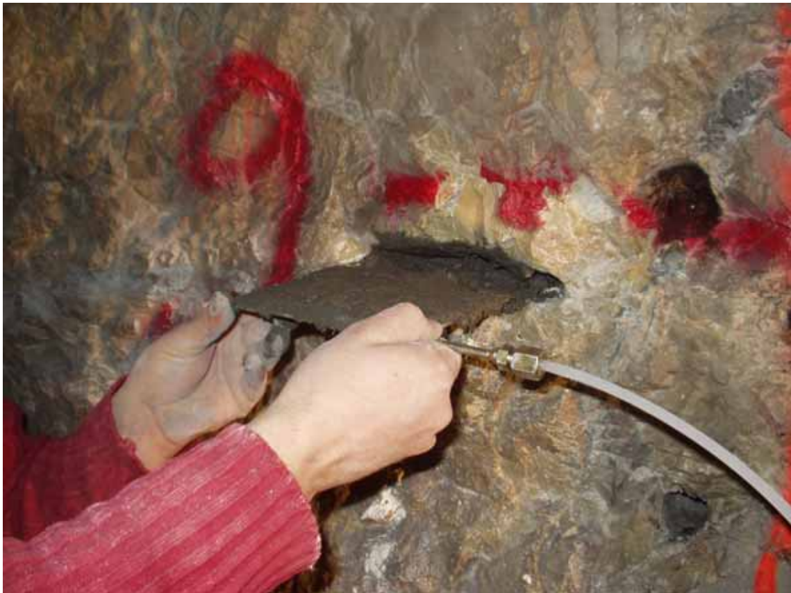
Installation of tangential pressure cell
