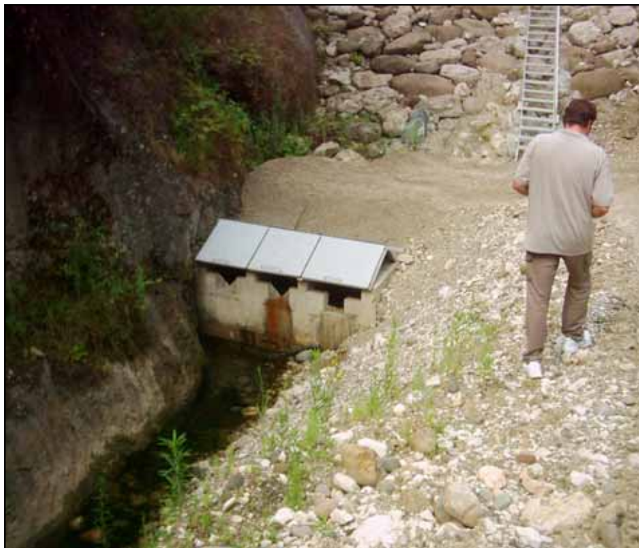
V-notch for leakage measurements
