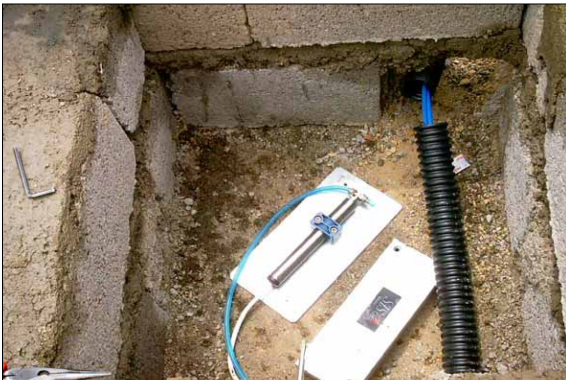
DSM hydraulic settlement system – embankment gauge
