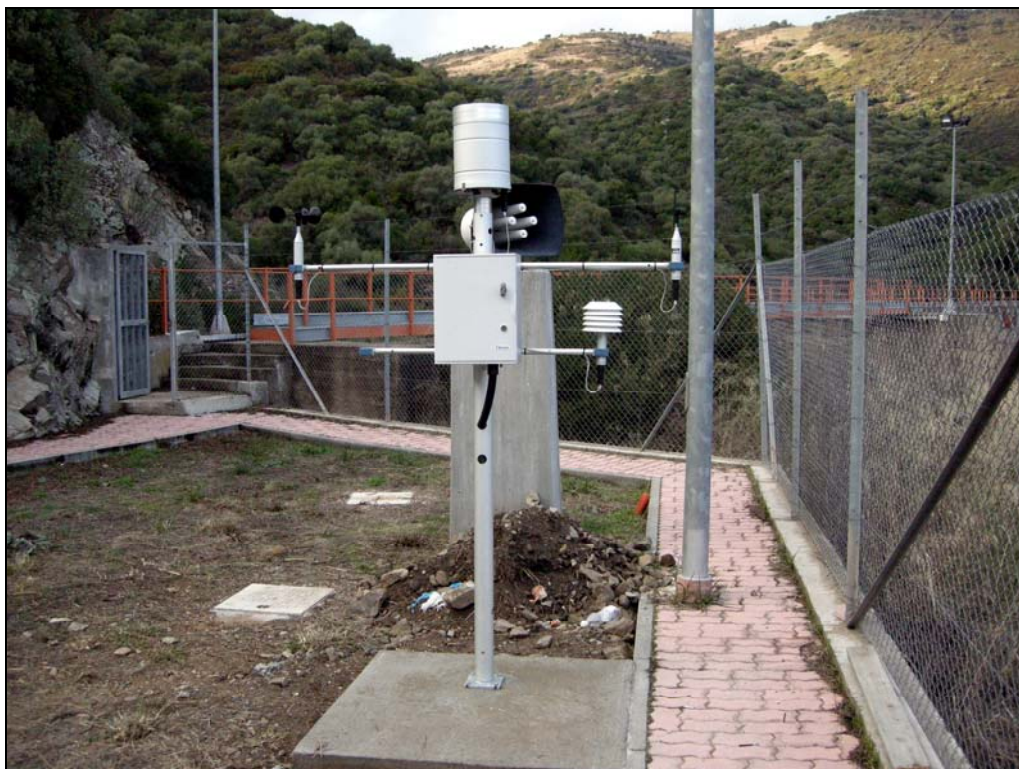
Installation of the meteorological station
