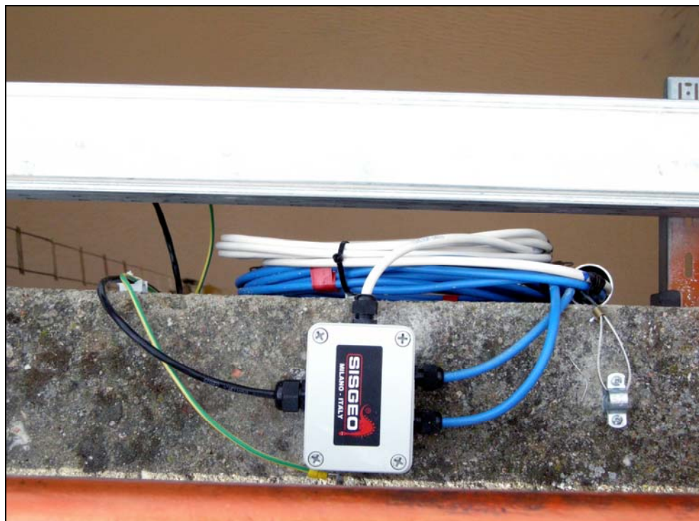
Installation of the reservoir water level trasducer and two termometers inside a inox conduit, all instruments connected to a OVP box.
