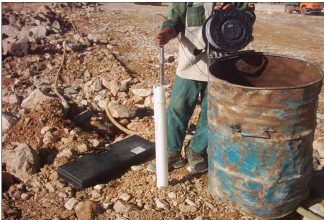
Test of inclinometer casing with dummy probe
