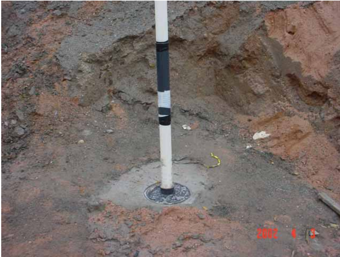
Combined inclinometer-settlement column and magnet ring within dam filling
