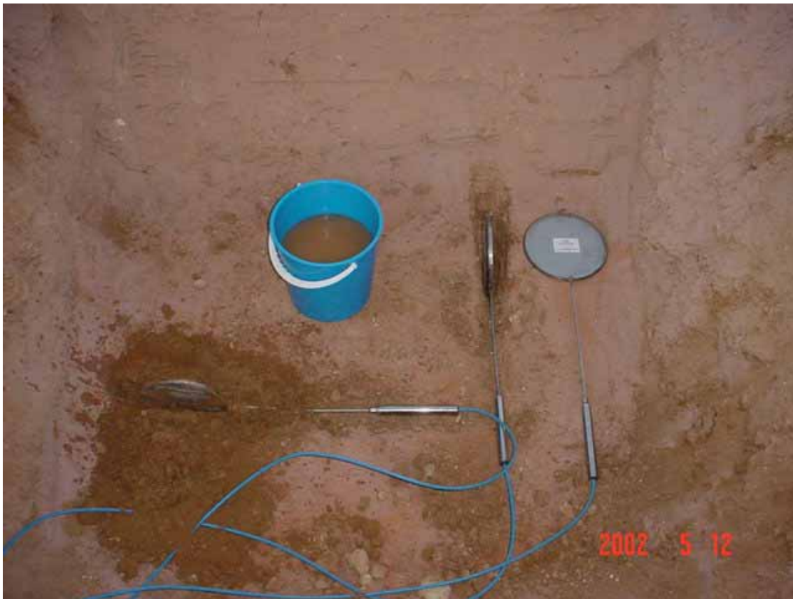
Earth pressure cells for 3D stress monitoring in the clay core
