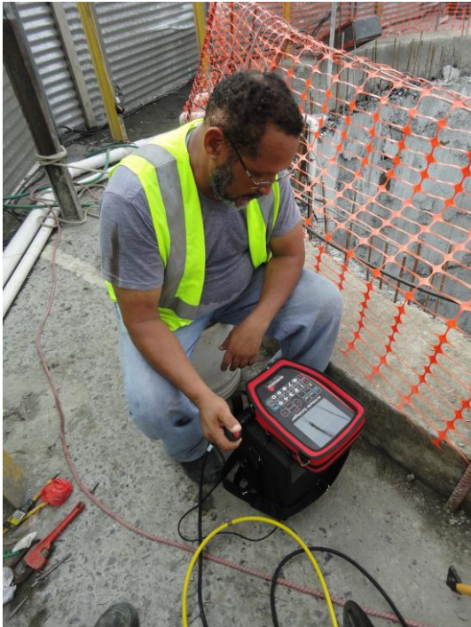
Inclinometer measurement with new Archimede readout
