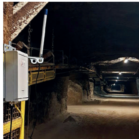
WR-Log installation in Varangéville Salines Mine - France
