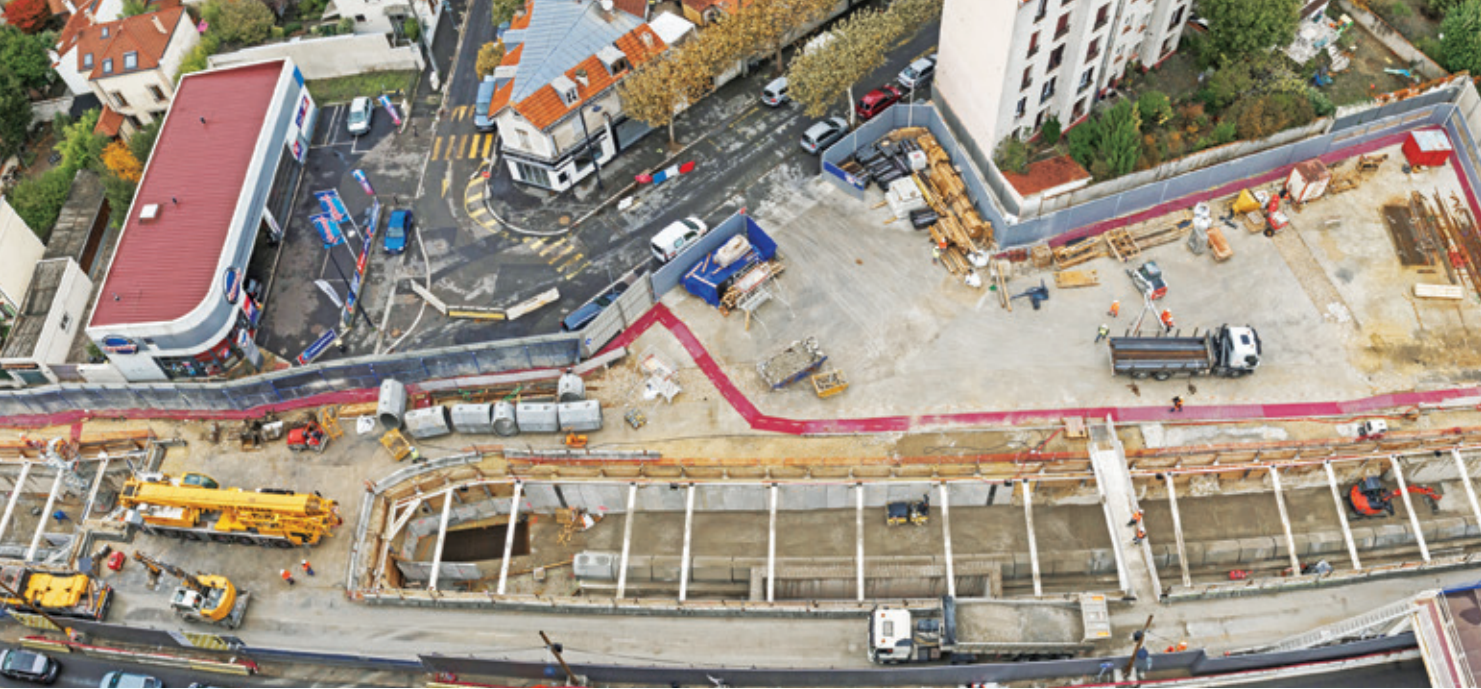
BH-Profile In Place Inclonometer head Thessaloniki Metro - Greece
