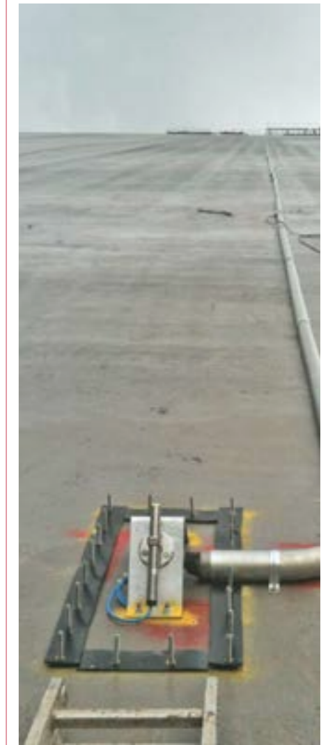
Submersible tilt meter installed on up-stream face of Sogamoso Dam - Colombia (190mt high)
