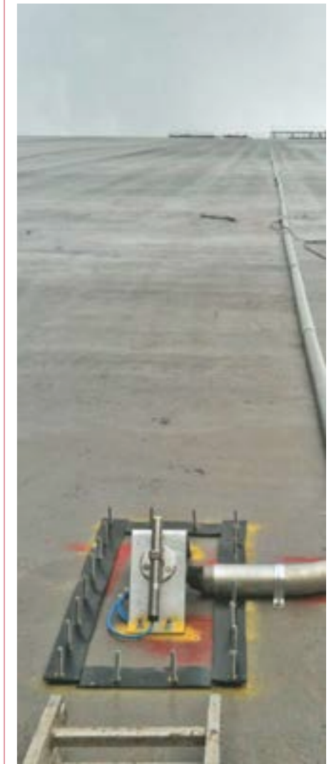
Submersible tilt meter installed on up-stream face of Sogamoso Dam - Colombia (190mt high)
