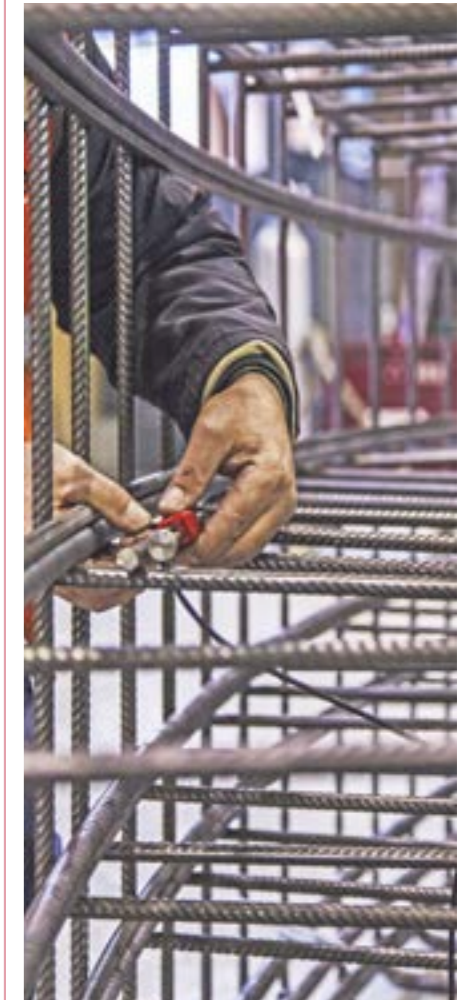
TELT - Tunnel Euralpin Lyon Turin, installation of VW strain gauges within TBM precast concrete element.
