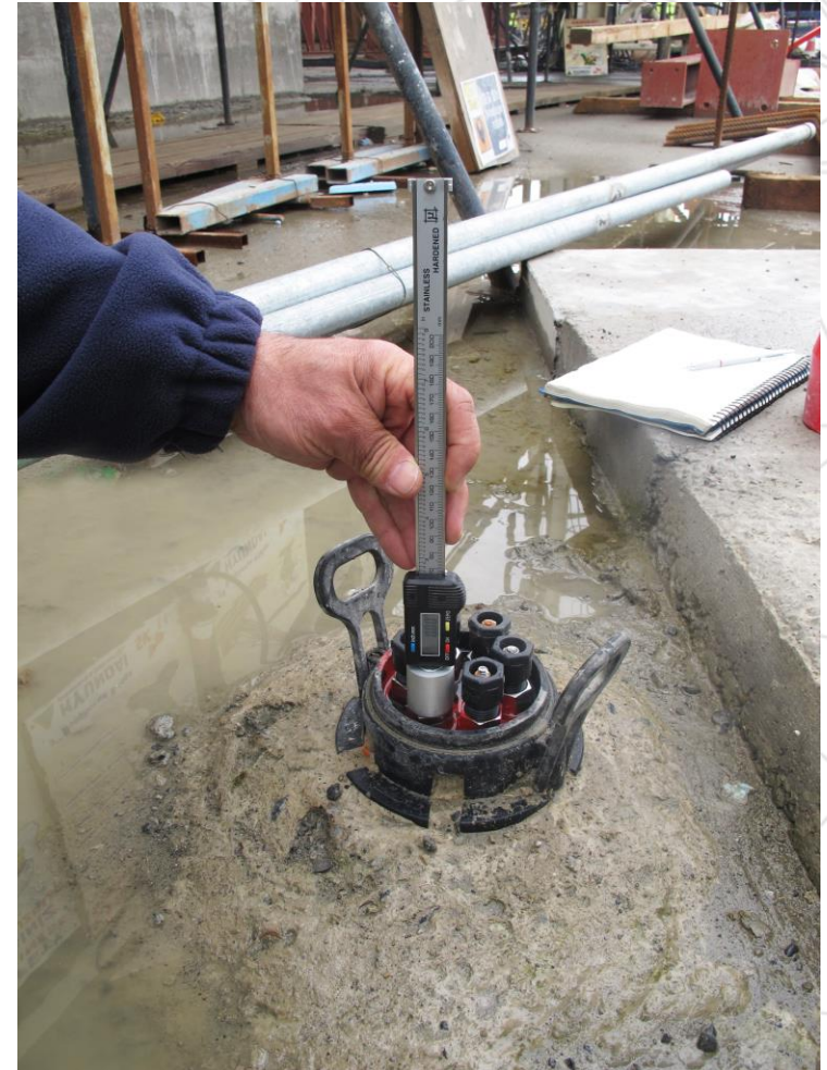
MPBX in dam lower tunnel
