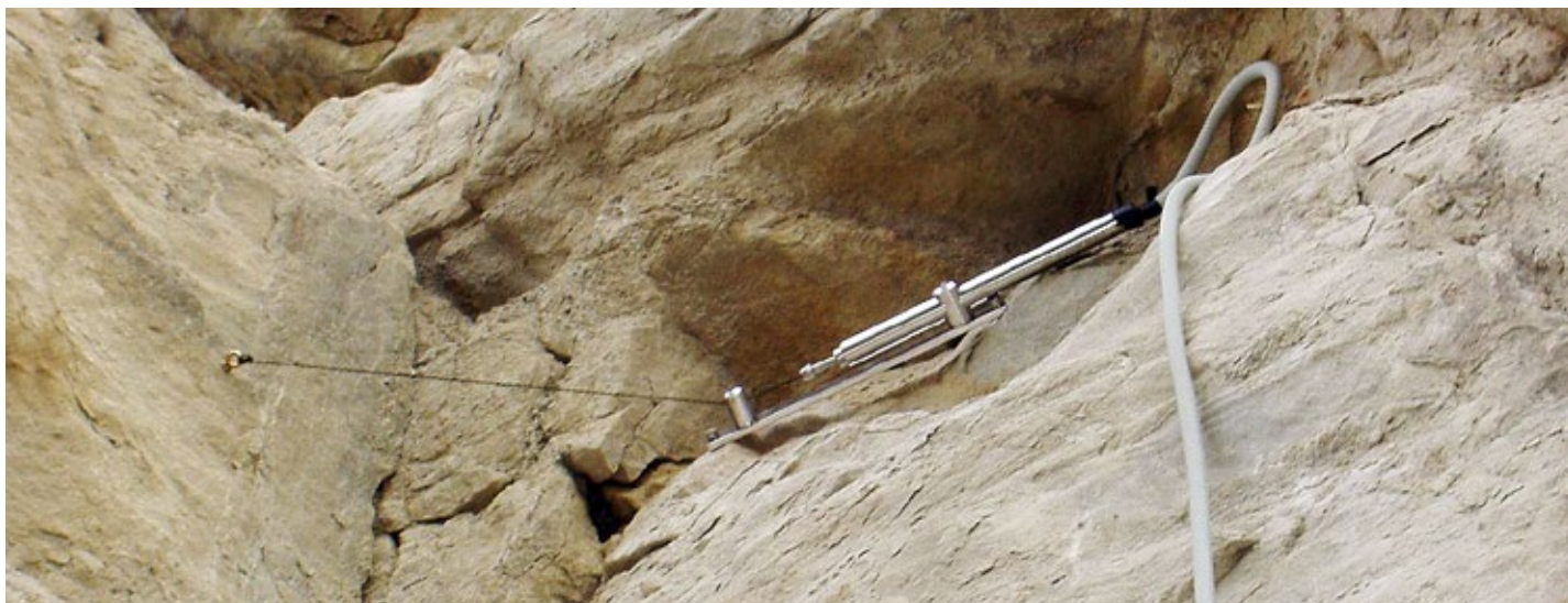
Electrical deformer installed on a rock fall
