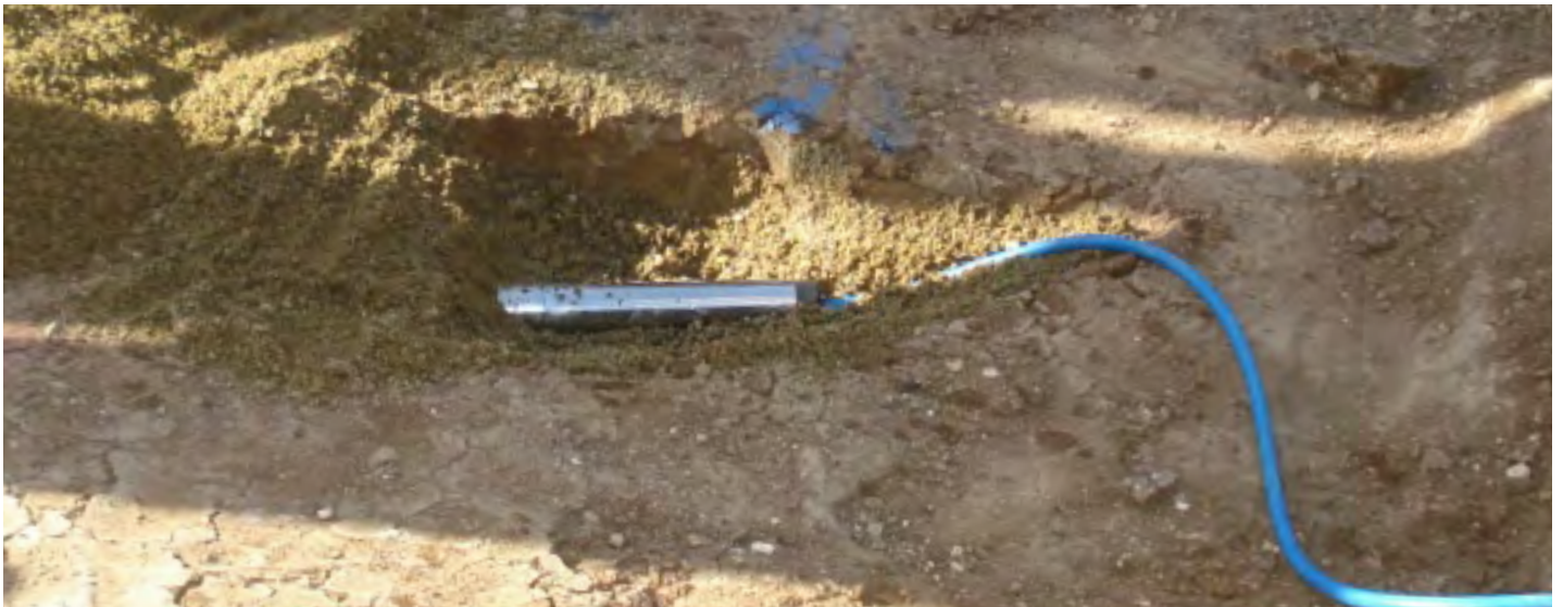
Vibrating wire piezometer in embankment dam foundation
