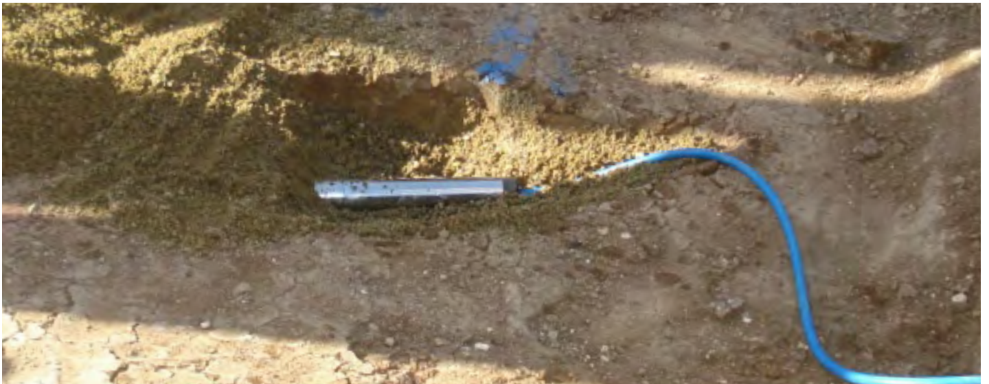
Vibrating wire piezometer in embankment dam foundation
