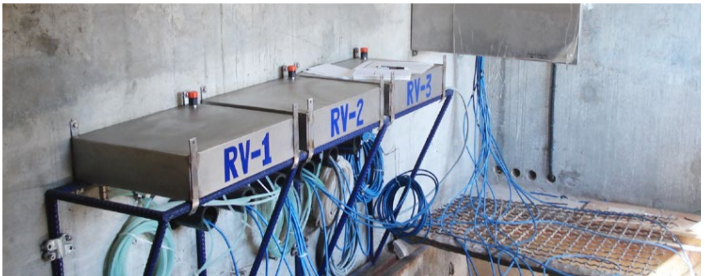
Reference vessels in Sogamoso HPP project, Colombia
