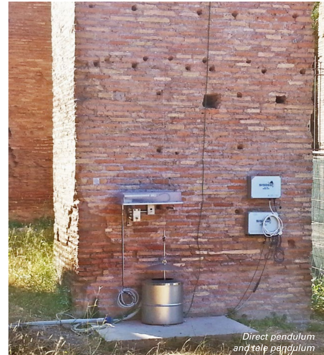
Digital tiltmeter installed on Maxentius Basilica
